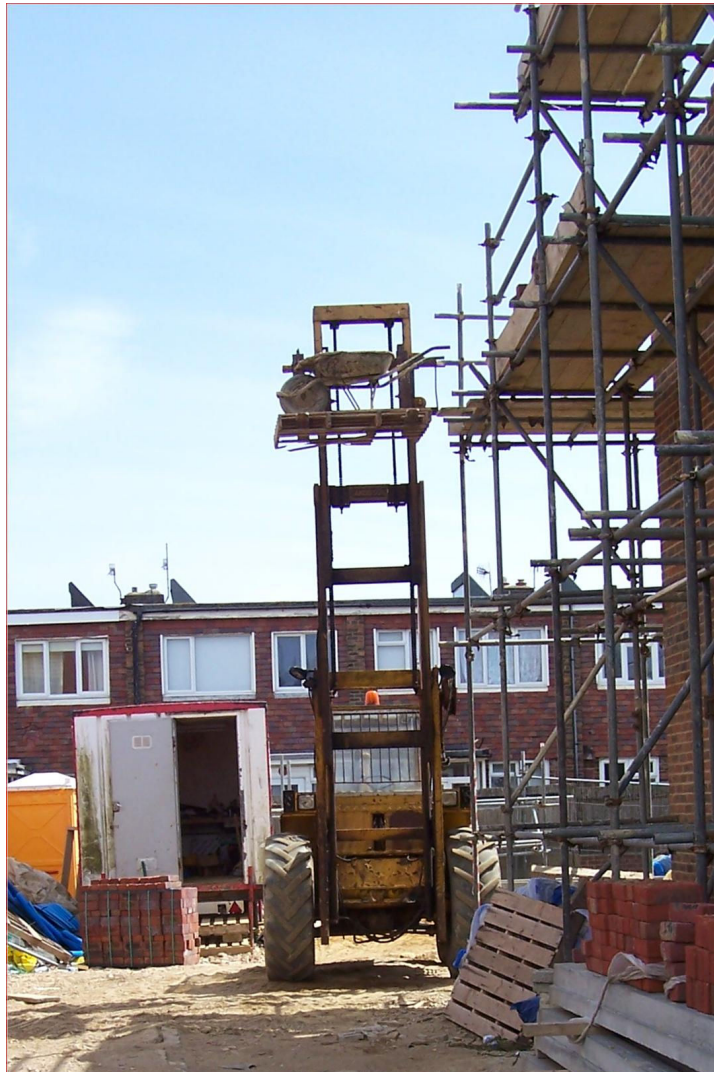
Inappropriate use of the forklift can cause falls from heights.
